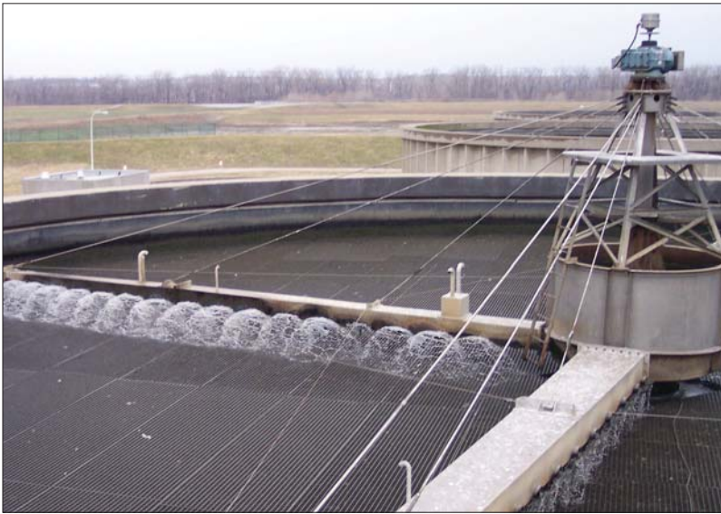
THIS IMAGE SHOWS ONE OF SEVERAL ON-SITE TRICKLING FILTERS.
